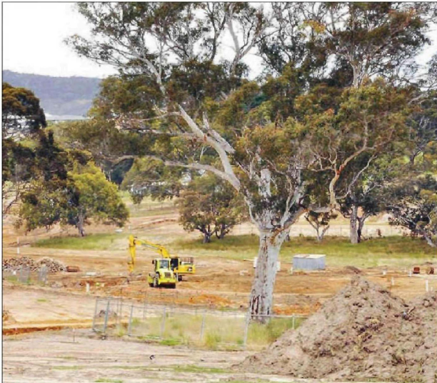
Contractors have started building the early infrastructure for a $100m Mt Barker housing estate that will focus on sustainability and energy security.
